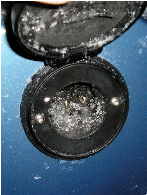
Iced receptacle on Unit #1982 (left)
