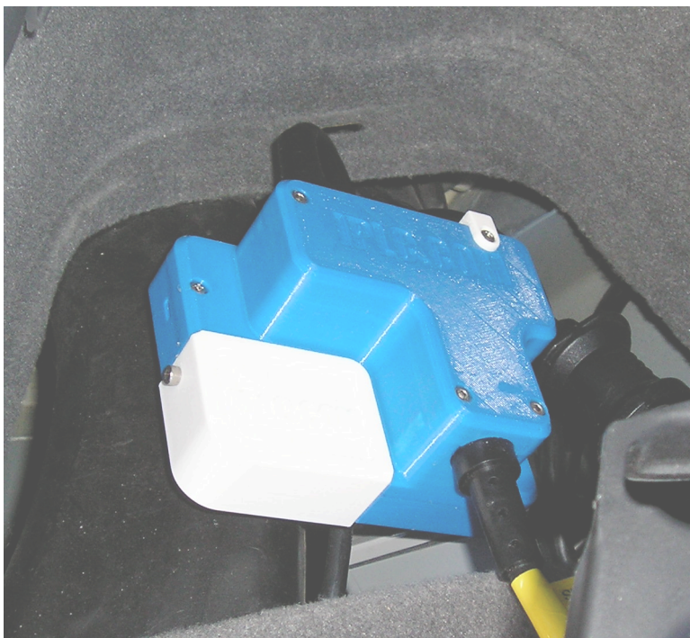
IPLC-PHEV PM2 Meter installed in Unit #1982
