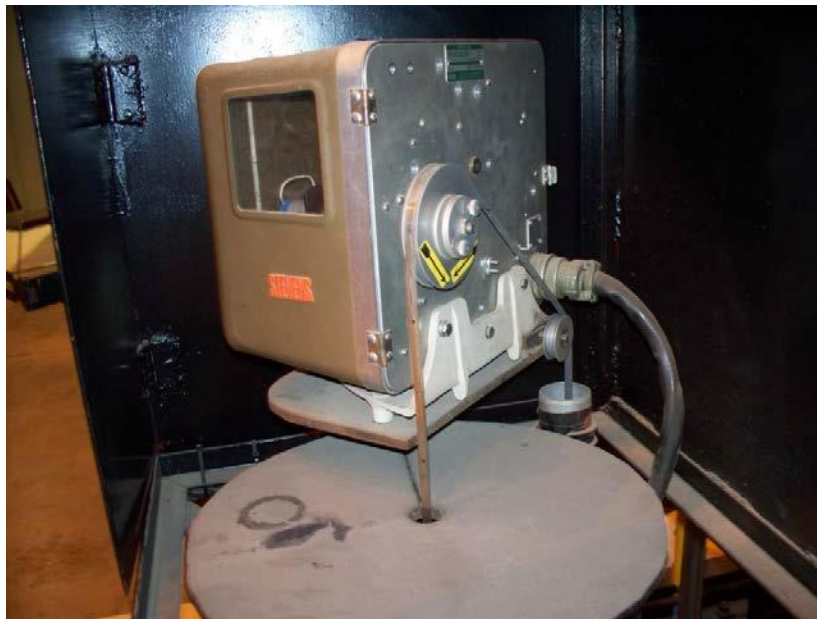
Tailrace Still-well Gauge
