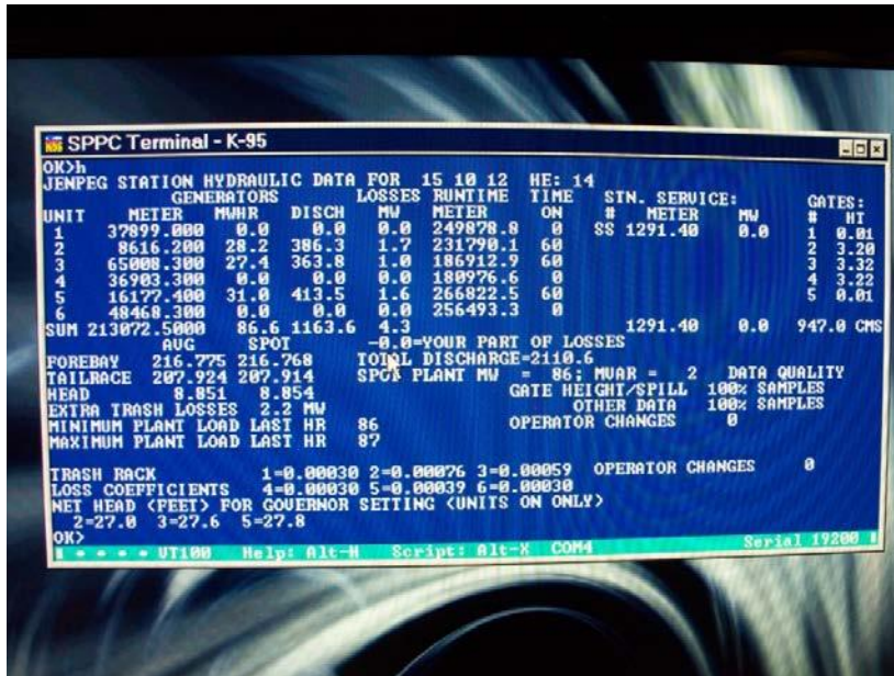
Screen Display of Stored Program Process Computer
