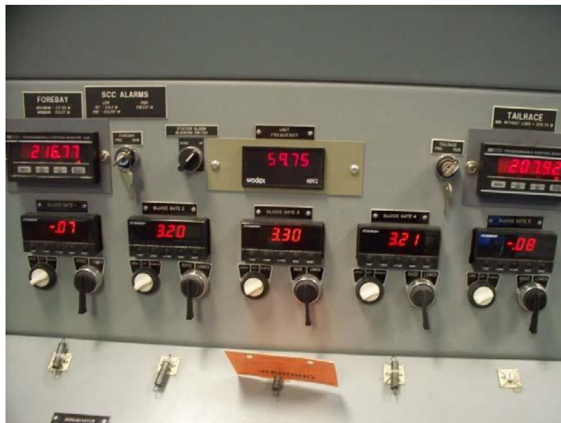
Control Room Digital Display of Forebay, Tailrace and Spillway Gate Positions
